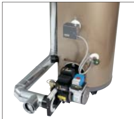
Closeup of burner and air intake boot.
